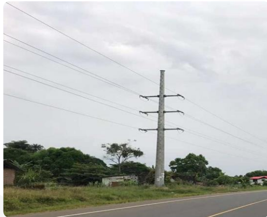
● 66 kV Line Paynesville
