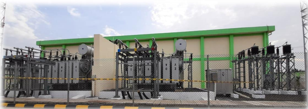
● Commissioning of GIS substation at, Monrovia, Liberia By His Excellency, President of Republic of Liberia Dr. George Manneh Weah
