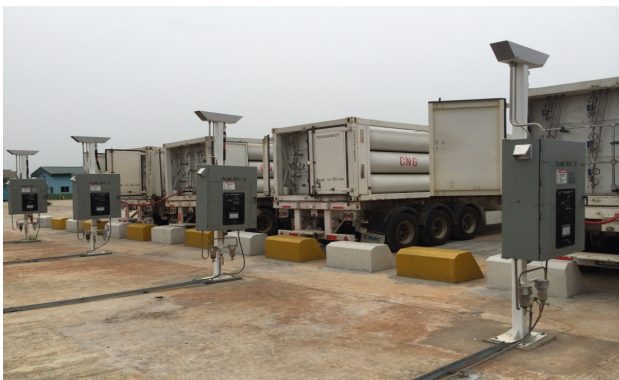
CNG TUBE SKID
